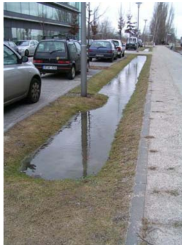
Figure 6 Trough infiltration system in Berlin, lacking vegetation (priority 7)
